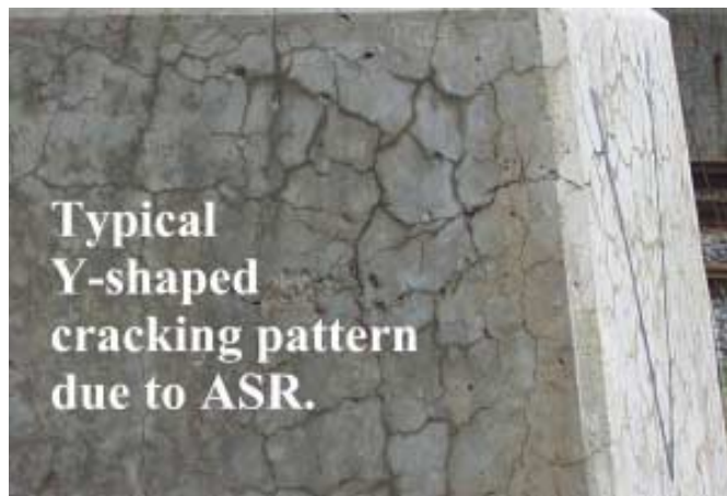
Fig. 3: Physical distress mechanisms of ASR include “Y-shaped” cracks as shown here
