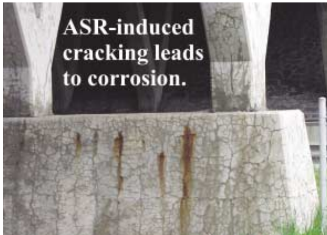
Fig. 2: As ASR progresses, the cracked concrete allows other distress mechanisms to occur, including corrosion of reinforcing steel
