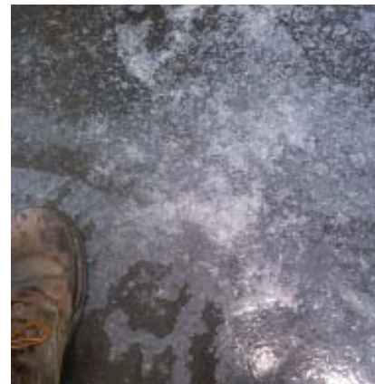
An excessively heavy application of sealer led to blushing followed by complete bond failure.
