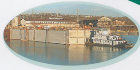
After construction of the Braddock Dam is completed, the capacity for traffic will be doubled
